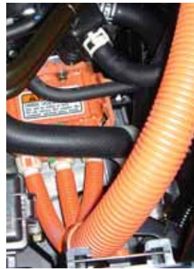
High-Voltage Cable Connection to Motor
