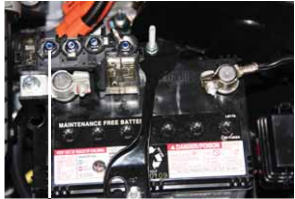
DC to DC Converter Cable Connection
